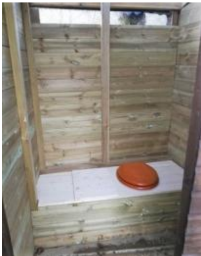
Interior of compost toilet
